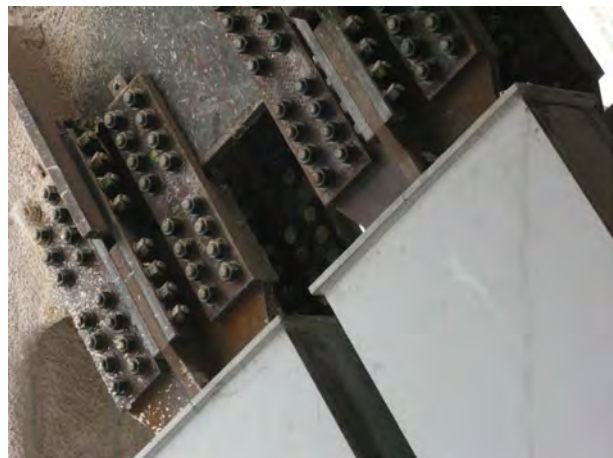
Figure 8. Quadruple BRBs bolted to gussets at upper connections. Note access to inner bolts.
