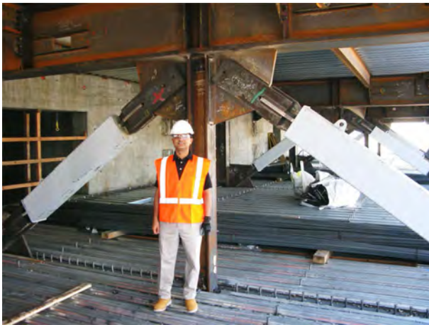
Figure 9. Single BRBs at middle outrigger use field welded splice plate connections. The red X shows a delayed connection.
